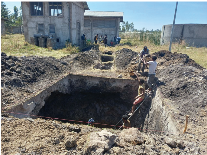
Drainage system construction at Derara Gorbe booster station, Awada Boricha Utility, Sidama Region
