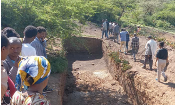
Figure 1: Source Catchment protection work at Ebo MVS, Raya Azebo woreda, Tigray Regional State
