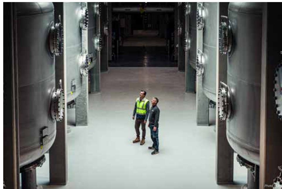
Congratulations to Greater Copenhagen Utility, who in September 2022 put one of their largest waterworks (the waterworks at Søndersø) back into operation after extensive modernisation.
