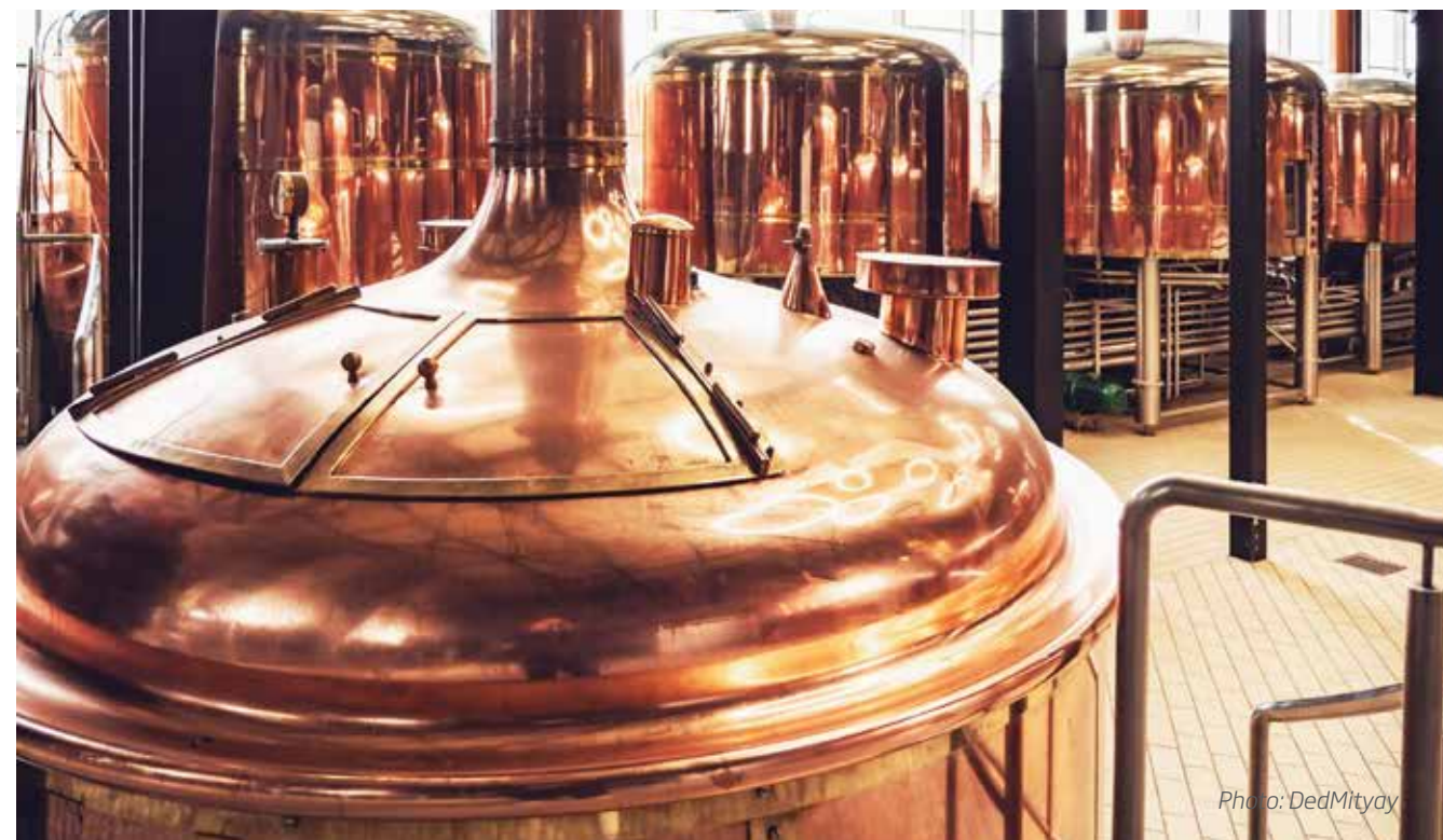
Copper tanks for beer fermentation and maturation.
